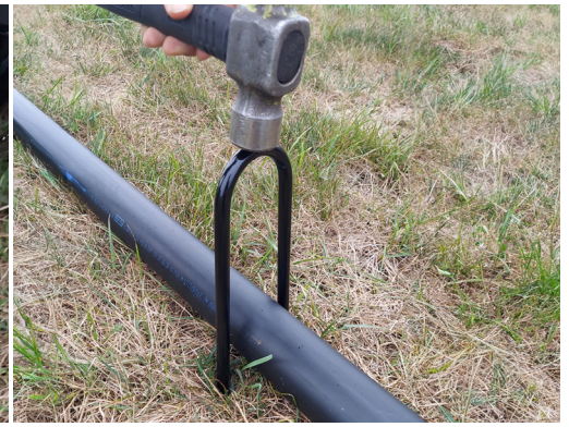
STEP 15 Straighten pipe and install U post halfway between hopper and front end of pipe
